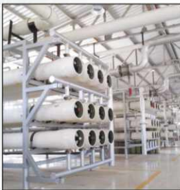
Industrial Ro. Plant
